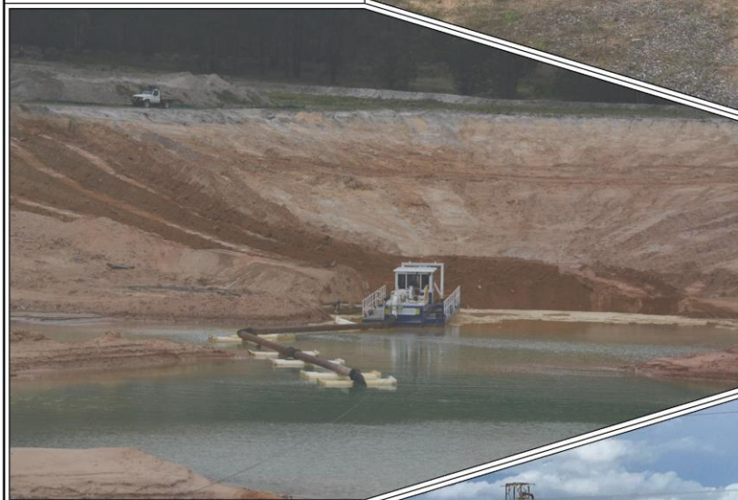
Plate 3: Dredge Pond - December 2017 Sand extraction within the Dredge Pond - Tinda Creek Quarry is a primarily 'wet' operation
