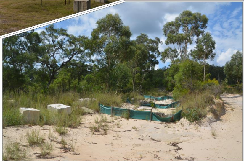
Plate 4: View of erosion sediment controls in the headwaters of Tinda Creek (Ref: E890F_086)
