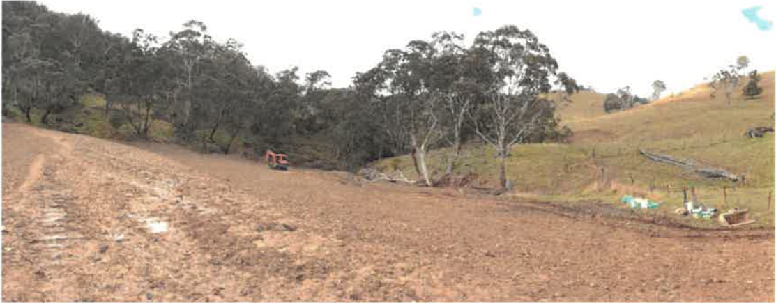
All materials were taken down to area for planting and Site was prepped – with help by ripper
