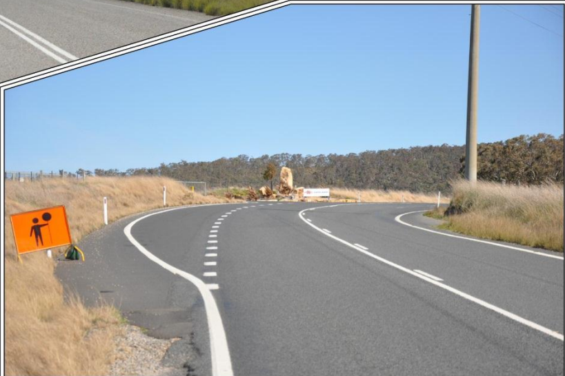
Plate 1.8: Deceleration lane on Jenolan Caves Road approaching the Quarry Entrance (Ref: E652P_063)
